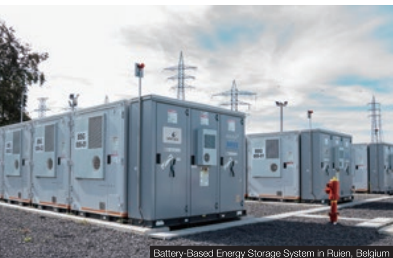
Battery-Based Energy Storage System in Ruien, Belgium
