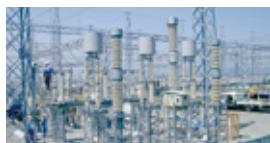
Japan Blocking coils (Line trap)
