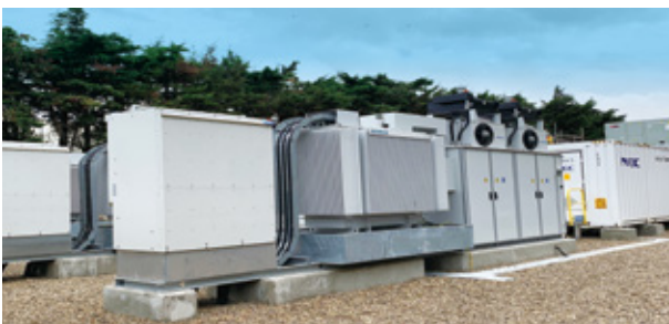
Storage batteries used in the Port of Tilbury Project in the United Kingdom
