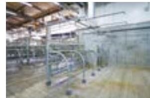
Berthing facility with misting system
