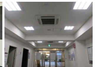
Plant upgraded with new LED lighting fixtures (Azuchi Plant)
