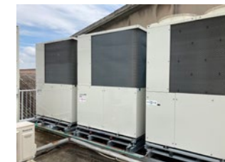
Renewal of GHP (Kyoto Plant)
