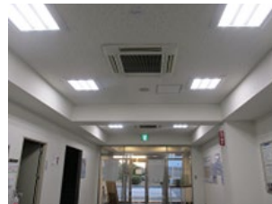
Conversion to LED lighting (Azuchi Plant)
