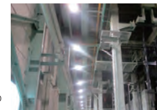
Plant upgraded with new LED lighting fixtures
