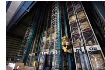
CAS PACK automated warehouse
