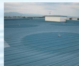
Rooftop sprinklers at Taiyo Chemical Industry Fujioka Plant
