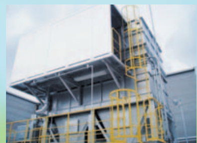
Exhaust gas and solvent treatment units
