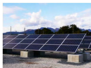
Hongo Photovoltaic Power Plant
