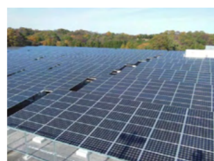
Elna Shirakawa Photovoltaic Power Plant
