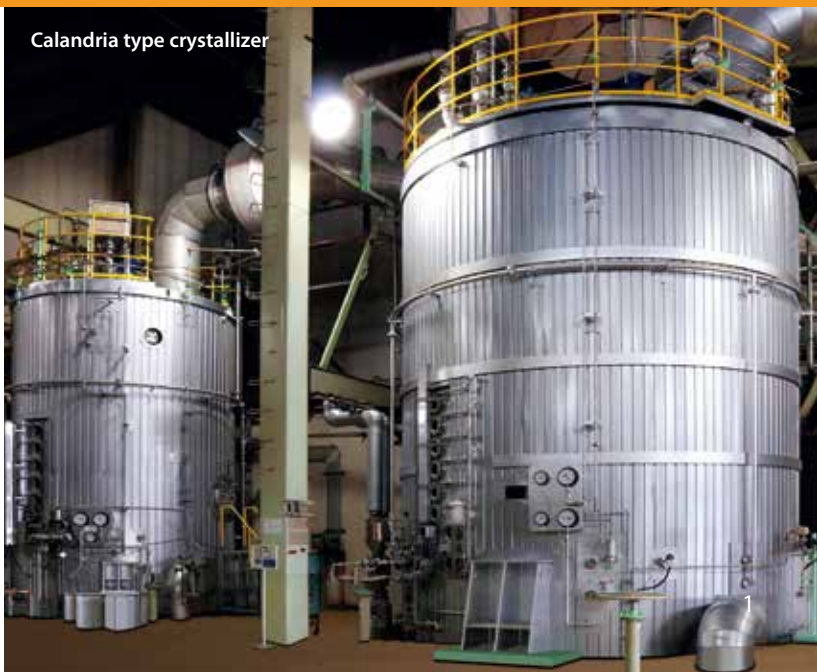
Sewage Sludge Dewatering and Drying system (demonstrated in B-DASH national project)
