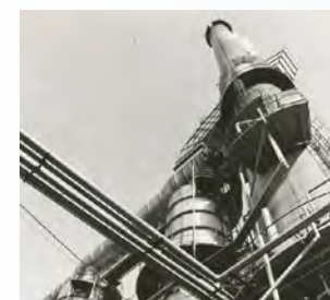
Exhaust desulfurization equipment
