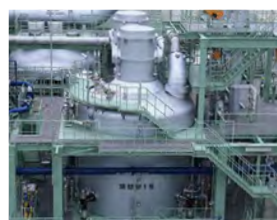
Sewage sludge incinerator
