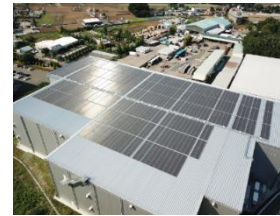
LogiSquare Niiza Solar Power Plant Power output: 898.56kW
