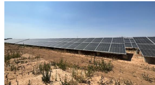
Solar power plant in Sabha, Mafraq (Jordan)
