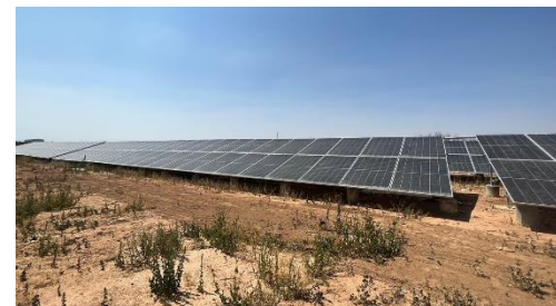
Solar power plant in Sabha, Mafraq (Jordan)
