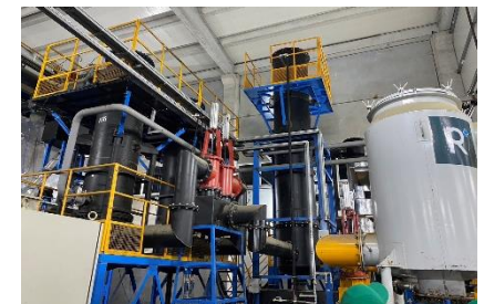
Biomass gasification power plant in operation in Goynuk, Bolu Province, northwestern Turkey
