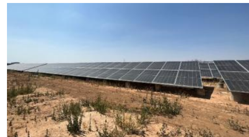
Solar power plant in Sabha, Mafraq (Jordan)
