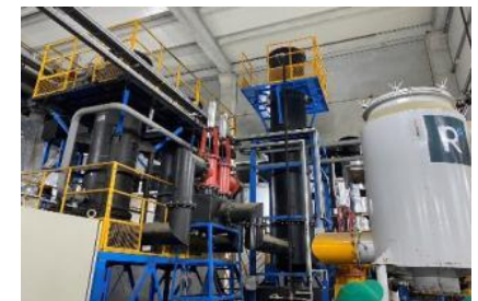
Biomass gasification power plant in Goynuk, Bolu Province in northwestern Turkey
