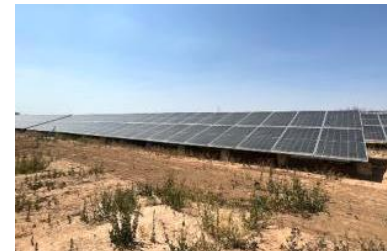
Solar power plant in Sabha, Mafraq (Jordan)
