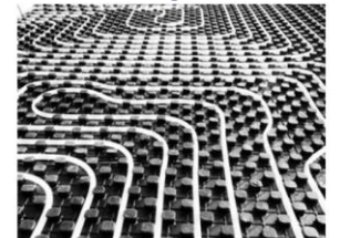
Under-floor heating pipes
