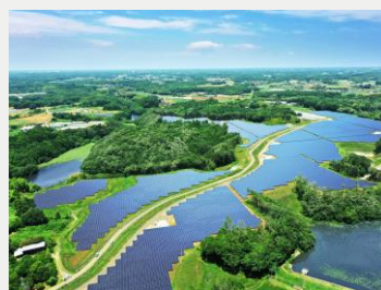
ReENE Namegata Solar Power Plant (Ibaraki) Rated capacity: 28MW (Operation started in FY2020)
