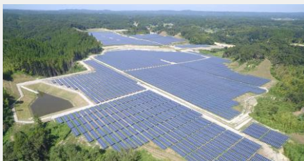
ReENE Chonan Solar Power Plant in Chiba : 24MW
