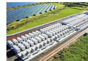
Storage batteries at Suzuran Kushiro cho Solar power plant
