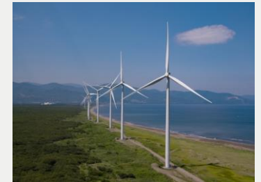
ReENE Zenibako Wind Power Plant (Hokkaido) Rated capacity: 34MW (Operation started in FY2019)
