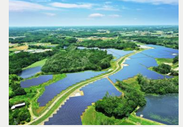
ReENE Namegata Solar Power Plant (Ibaraki) Rated capacity: 28MW (Operation started in FY2020)
