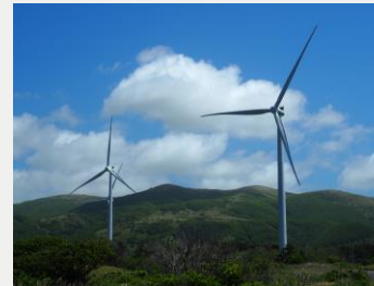
ReENE Matsumae Wind Power Plant (Hokkaido) Rated capacity: 41MW (Operation started in 2019)
