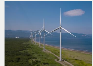
ReENE Zenibako Wind Power Plant (Hokkaido) Rated capacity: 34MW (Operation started in 2019)
