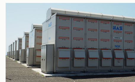
Utilizing a storage battery system for the stable supply of electricity
