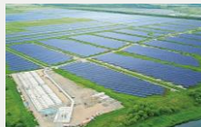
ReENE (Solar power generation facilities)
