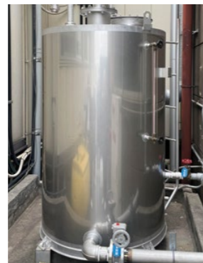
A water tank for a steam boiler at the Higashi-Osaka Plant of Initio Foods
