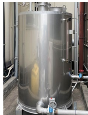
A water tank for a steam boiler at the Higashi-Osaka Plant of Initio Foods
