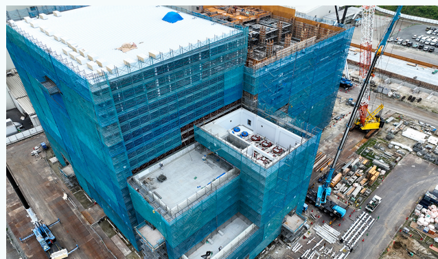
Nisshin Flour Milling Inc.'s Mizushima Plant (under construction aiming for start of operation around May 2025)
