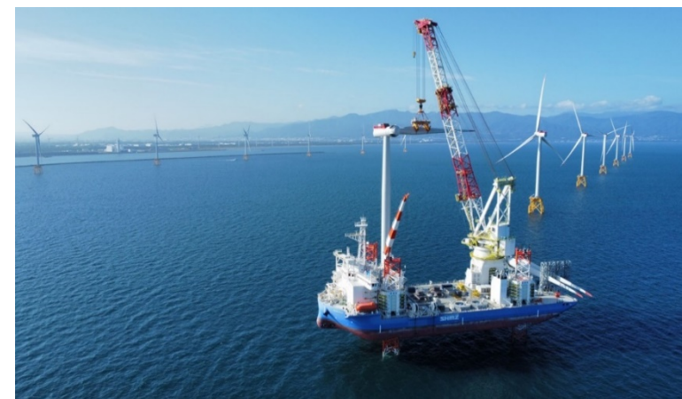
Ishikari Bay New Port Offshore Wind Farm Constructed by our self-propelled SEP vessel "BLUE WIND"
