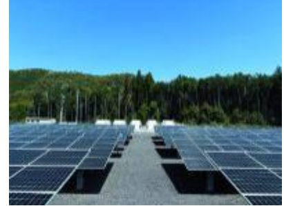
Isa Battery Energy Storage System with Solar Power Plant
