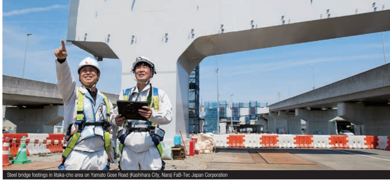
Steel bridge footings in Iitaka-cho area on Yamato Gose Road (Kashiwara City, Nara) FaB-Tec Japan Corporation
