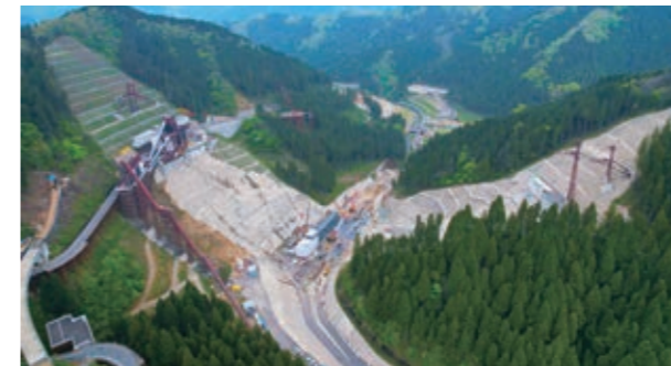
Asuwa River Dam construction as seen from upstream (Ikeda Town, Imadate District, Fukui)
