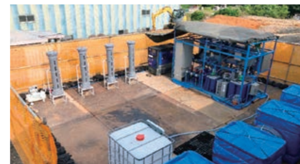
Organic fluorine compound (PFAS) sewage purification demonstration facility (Okinawa, Japan)
