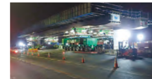
Multi-axle transporter installation between P1 and P2 of Ohibashi-Nishi Viaduct (commissioned by the Chugoku Regional Development Bureau, Ministry of Land, Infrastructure, Transport and Tourism)
