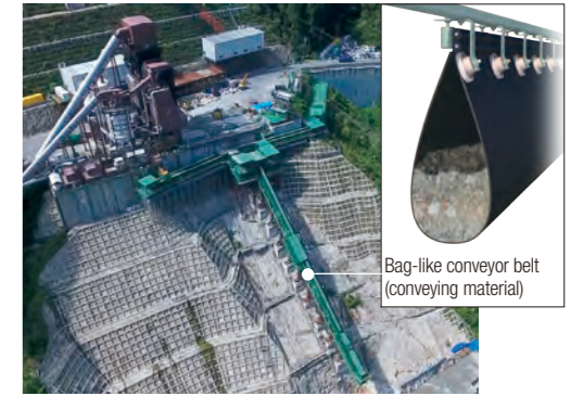
SC premium belt conveyor installation (Ikeda-cho, Imadate-gun, Fukui Prefecture)
