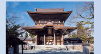
2023 Preservation and Repair Work on Romon Gate of Aso Shrine Rebuilt the gate, which was completely destroyed in the 2016 Kumamoto earthquake. The materials were repaired wherever possible and reused.
