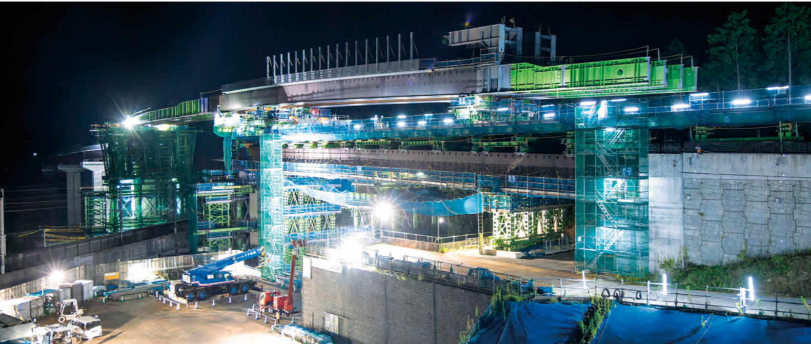
Construction of the Kojo overbridge No. 2 in the Shin-minamata Station precincts and three other works (Minamata City, Kumamoto Prefecture), with bridge erection across the Kyushu Shinkansen using the launching erection method
