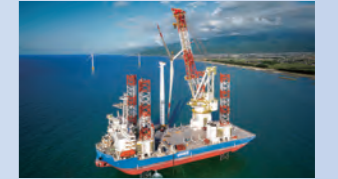
2023 Nyuzen Offshore Wind Power Farm Constructed using our self-propelled SEP vessel BLUE WIND. An EPC project that manages design, procurement, and construction as a single package.
