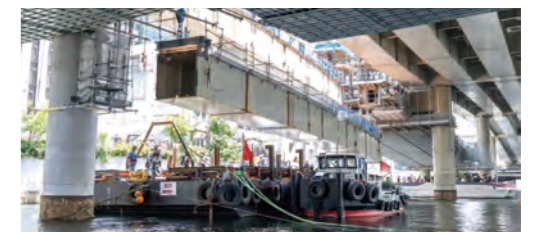
Removing a steel bridge beam by suspending and lowering it with the use of a barge (Chuo Ward, Tokyo)
