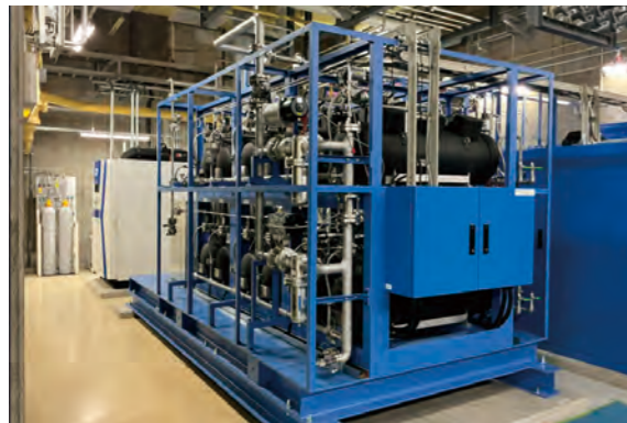
Hydro Q-BiC hydrogen storage alloy tank (inside the Aomi Minami Plant of Tokyo Rinkai Heat Supply Corporation, Tokyo)
