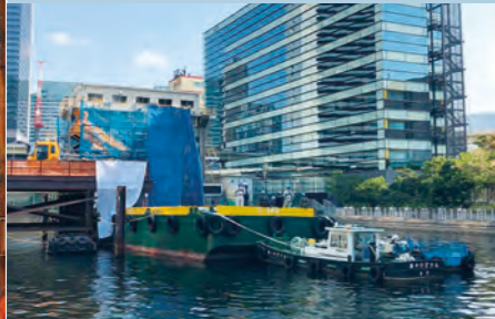
A temporary pier enabled transportation of excavated soil away from site by boat
