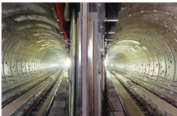
TAIWAN TAOYUAN INTERNATIONAL AIRPORT ACCESS MRT SYSTEM CONSTRUCTION PROJECT - CONTRACT NO. CA450A CIVIL CONSTRUCTION, Taiwan
