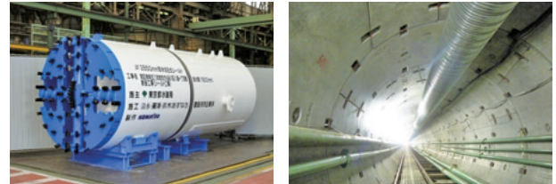
Installing a new water pipe from the area of Konan 5-chome in Tokyo s Minato Ward to Yashio 1-chome in Shinagawa Ward
