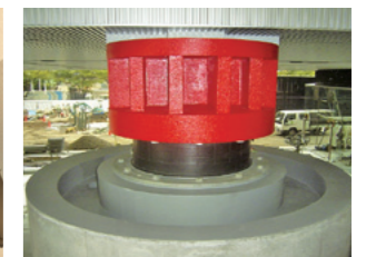
Seismic-isolation equipment at the Shimizu Institute of Technology
