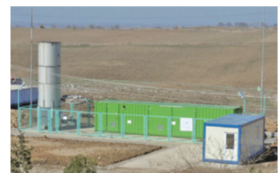
Methane gas collection facility in Uzbekistan
