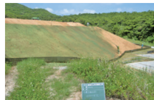
Sloping surfaces covered with grass seed and soil at the Gima Dam site
