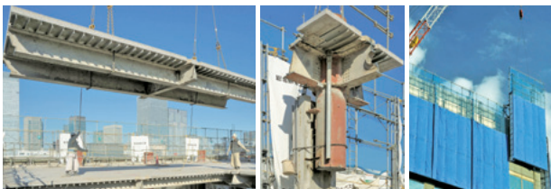
Separating a building into blocks (two photos at left) and lowering a block to the ground using a crane (photo at right)
