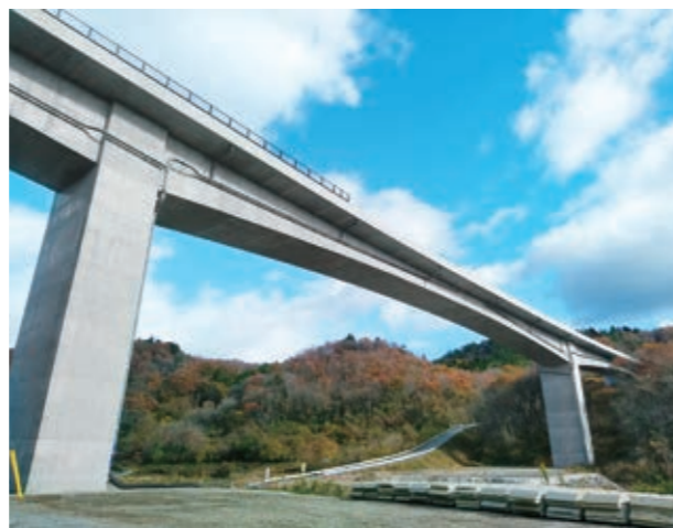
Sharaku was formally adopted for the first time in Japan Tohoku Chuo Expressway Higashinegawa Bridge (Tohoku Regional Development Bureau, Ministry of Land, Infrastructure, Transport and Tourism)
