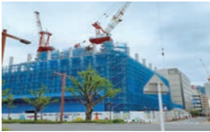
Nagoya Marunouchi 1-chome plan utilizing PC structural framework in exterior design (Nagoya City, Aichi)
