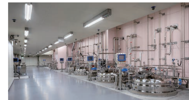
Lotion Manufacturing Room at Shiseido Osaka-Ibaraki Plant (Ibaraki City, Osaka)
