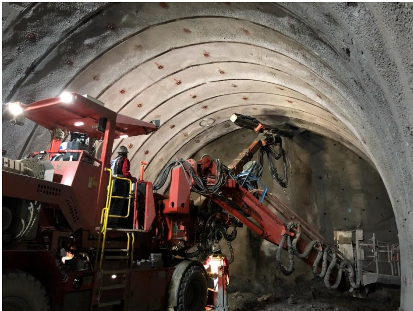
Blast Master Operation Status
