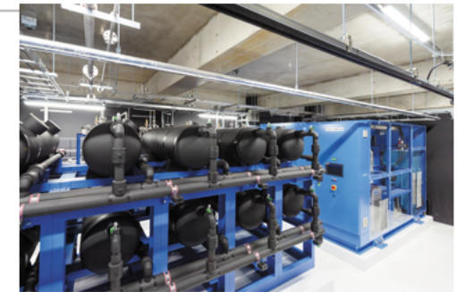
Hydro Q-BiC, hydrogen energy utilization system in a building
