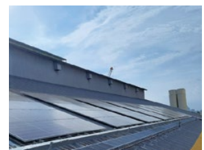
Solar power generation equipment Phrapradaeng Plant (Thailand, Nisshin-STC Flour Milling)
