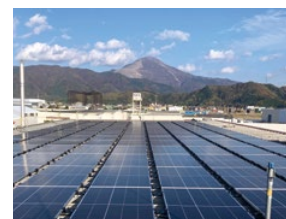
Solar power generation equipment (on-site PPA method) Nagahama Plant (Oriental Yeast)
