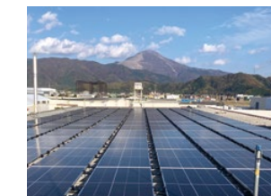
Solar power generation equipment (on-site PPA method) Nagahama Plant (Oriental Yeast)
