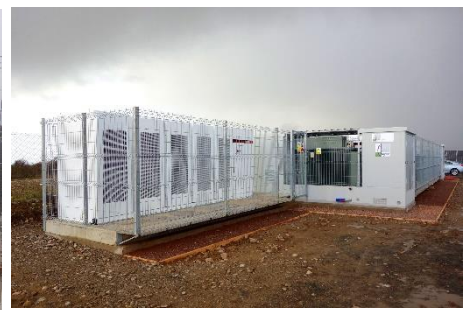
Battery system overview
