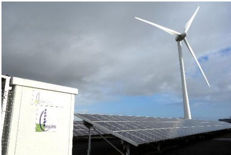
Project site along with Wind and Solar.
