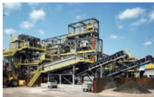
An on-site soil treatment plant (high-performance equipment capable of handling small-scale cases of soil pollution)
