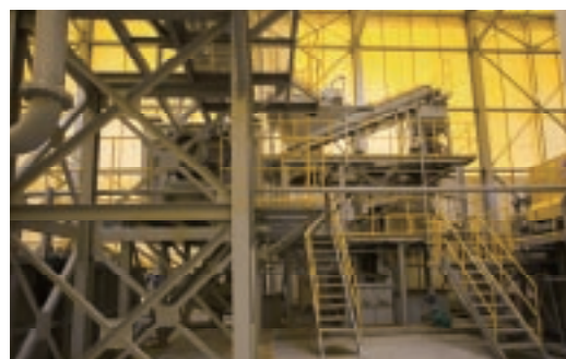
Remediation equipment in a treatment plant for dioxin-contaminated soil
